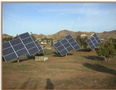
Solar panels rotate to track the Sun
