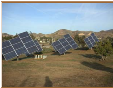
Solar panels rotate to track the Sun
